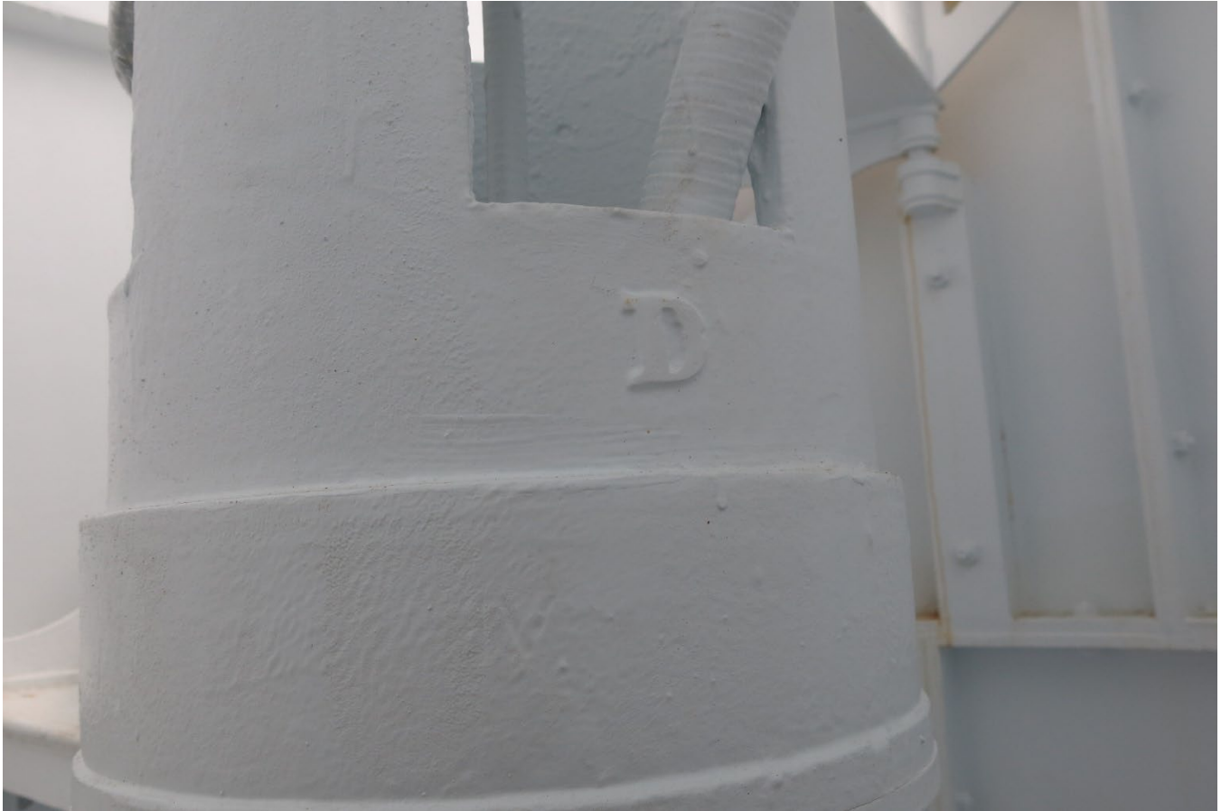
Photo 11. Example of lettered labeling on drop tube construction visible from the interior. (FL_Lee_SanibelLighthouse_11).
