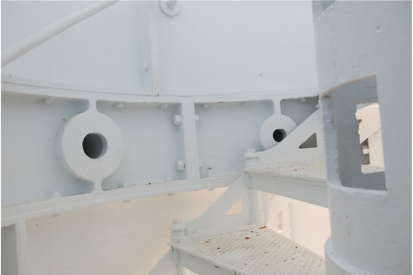
Photo 10. Example of plate assembly of the central cylinder visible from the interior walls. (FL_Lee_SanibelLighthouse_10).
