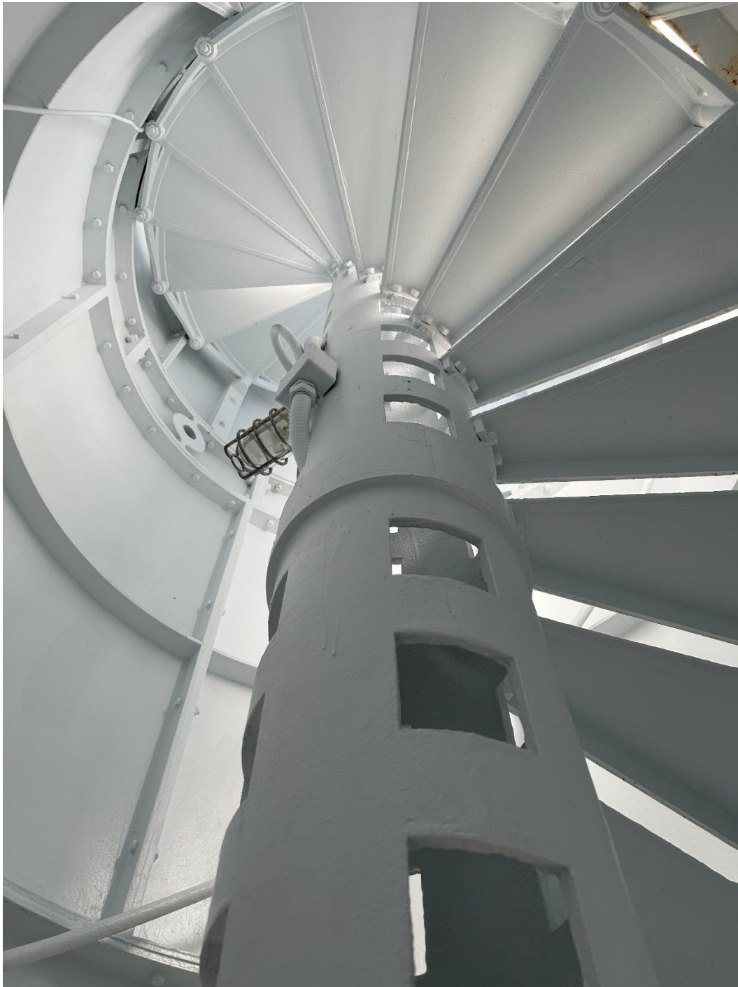
Photo 8. Looking upward within the central cylinder with stairs wrapping around the drop tube. (FL_Lee_SanibelLighthouse_08).
