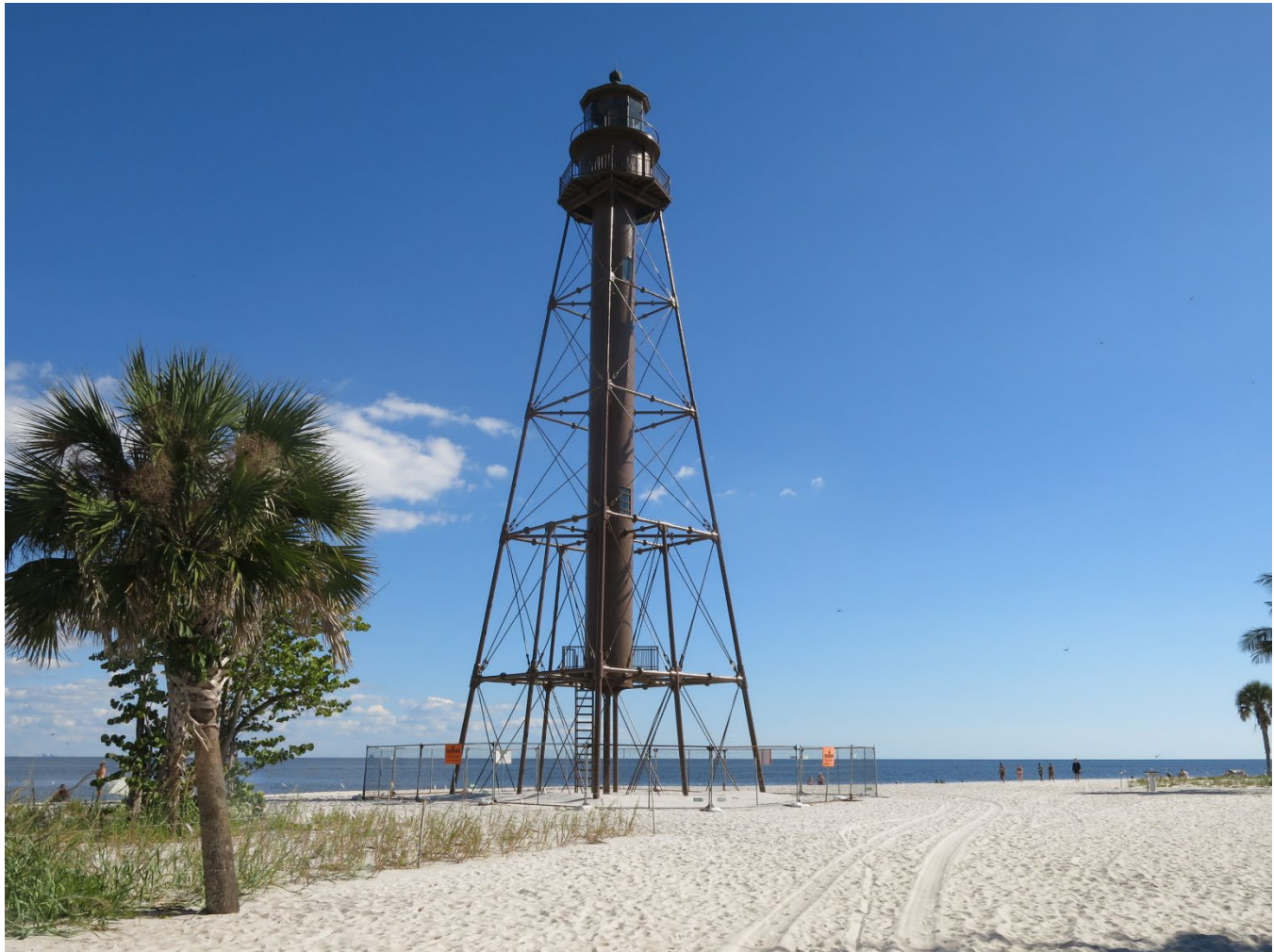
Photo 1. Setting of the Sanibel Lighthouse in 2025 following Hurricane Ian. Facing south. (FL_Lee_SanibelLighthouse_01).
