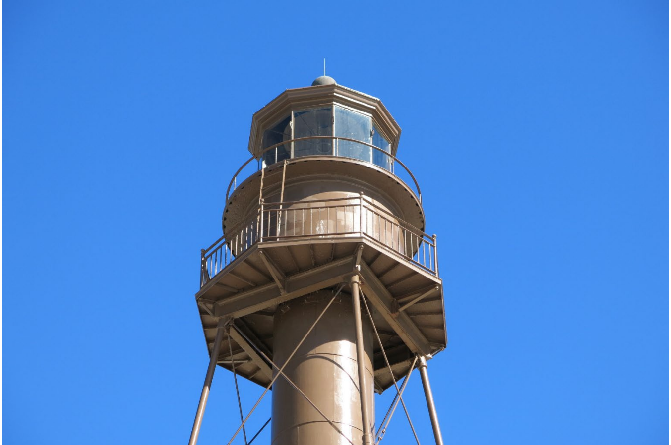
Photo 17. Exterior view of the watch room and lantern room with the exterior ladder leading between the watch room gallery and the lantern room gallery visible. Facing north. (FL_Lee_SanibelLighthouse_17).
