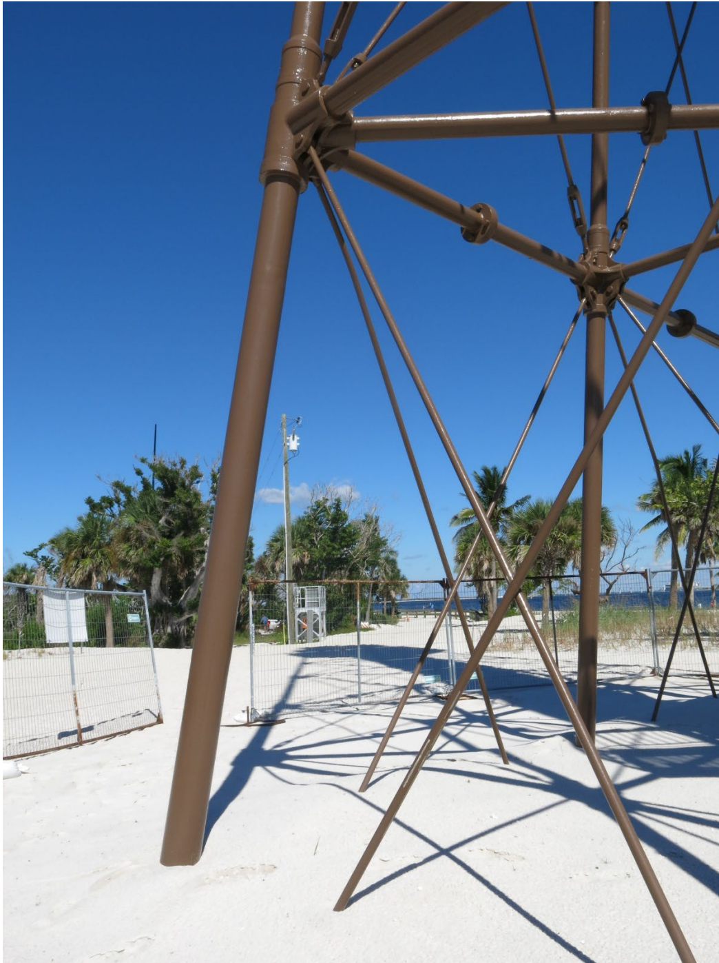
Photo 21. Replacement southwest support column manufactured to match the original columns, facing north. (FL_Lee_SanibelLighthouse_21).
