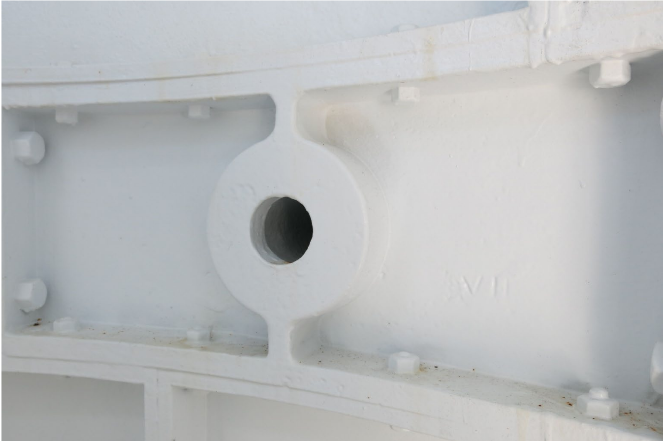
Photo 9. Example of plate assembly of the central cylinder visible from the interior walls. (FL_Lee_SanibelLighthouse_09).
