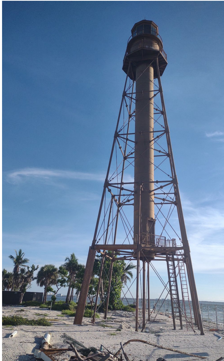
Photo 20. The Sanibel Lighthouse with temporary wooden leg installed and surrounded by debris following Hurricane Ian in 2022. Facing northeast. Photo taken by Kim Ruiz in August 2023. (FL_Lee_SanibelLighthouse_20).
