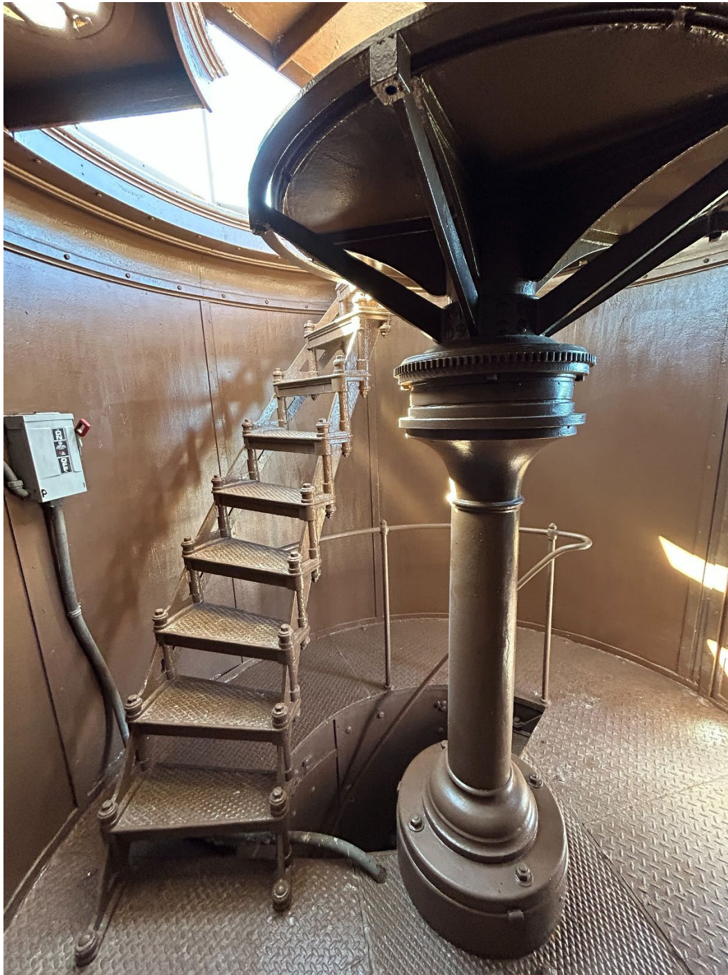
Photo 13. Interior view of the watch room with secondary stairs to lantern room and remnants of the rotator pedestal which supported the original lens. (FL_Lee_SanibelLighthouse_13).
