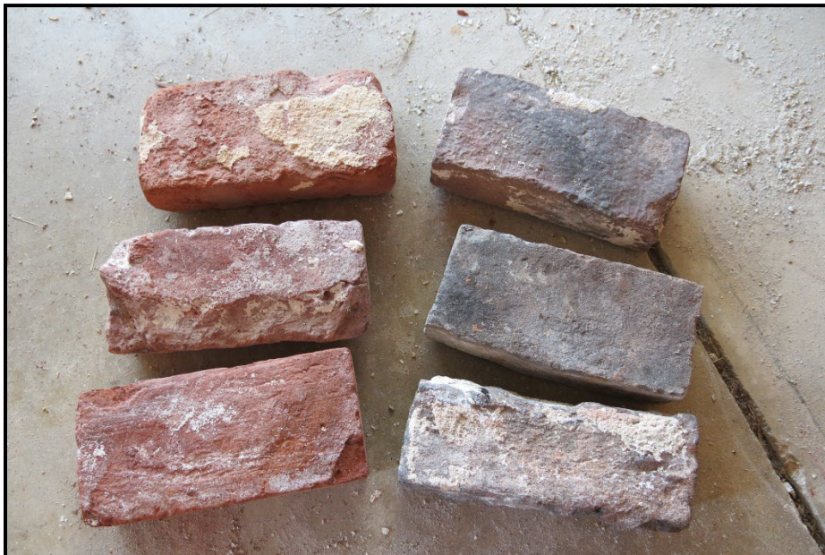
Photo 12. Three weathered examples of face brick (plain) (left) and face brick (charred) (right).
