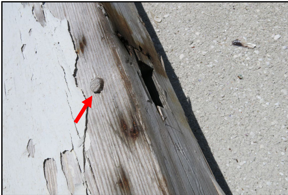
Photo 19. An example of a partially intact mortise and tenon joint along the top of the wooden girder. The rectangular cavity to the right is the mortise and the cylindrical wooden peg to secure the tenon (broken off) is visible to the left and indicated by the red arrow.
