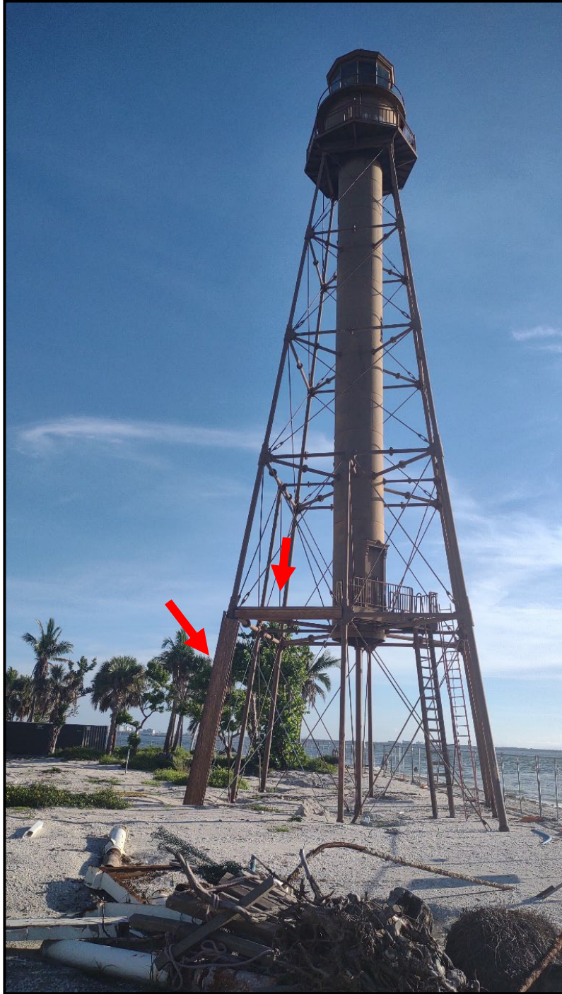
Photo 3. A photograph of the Sanibel Lighthouse following Hurricane Ian and prior to restoration work. Temporary wooden supports were installed and are indicated by the red arrows. Photo taken by Kim Ruiz, City of Sanibel Principal Planner, in August 2023.
