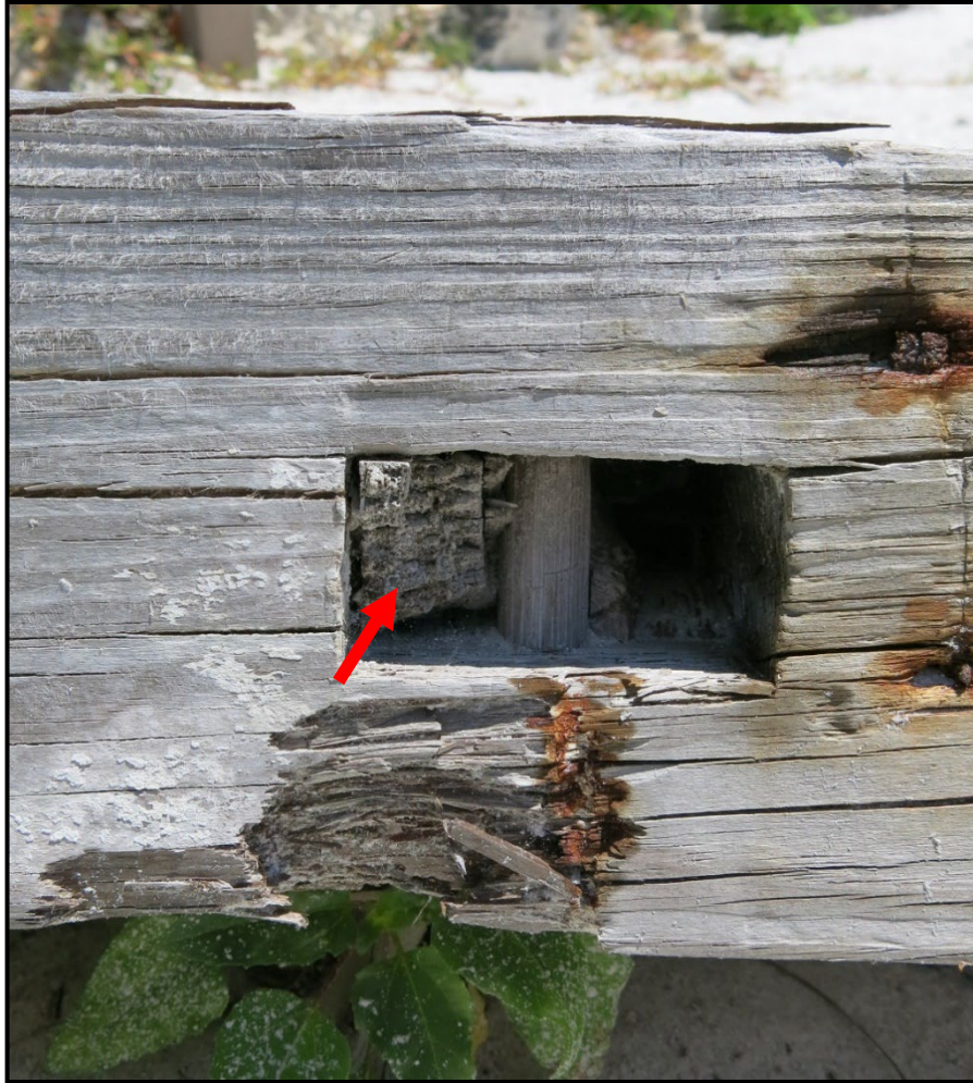
Photo 20. An example of a partially intact mortise and tenon joint along the top of the wooden girder. The rectangular cavity is the mortise, and it is bisected by a cylindrical wooden peg to secure the tenon. The tenon has broken off and only a small segment remains within the mortise (red arrow).
