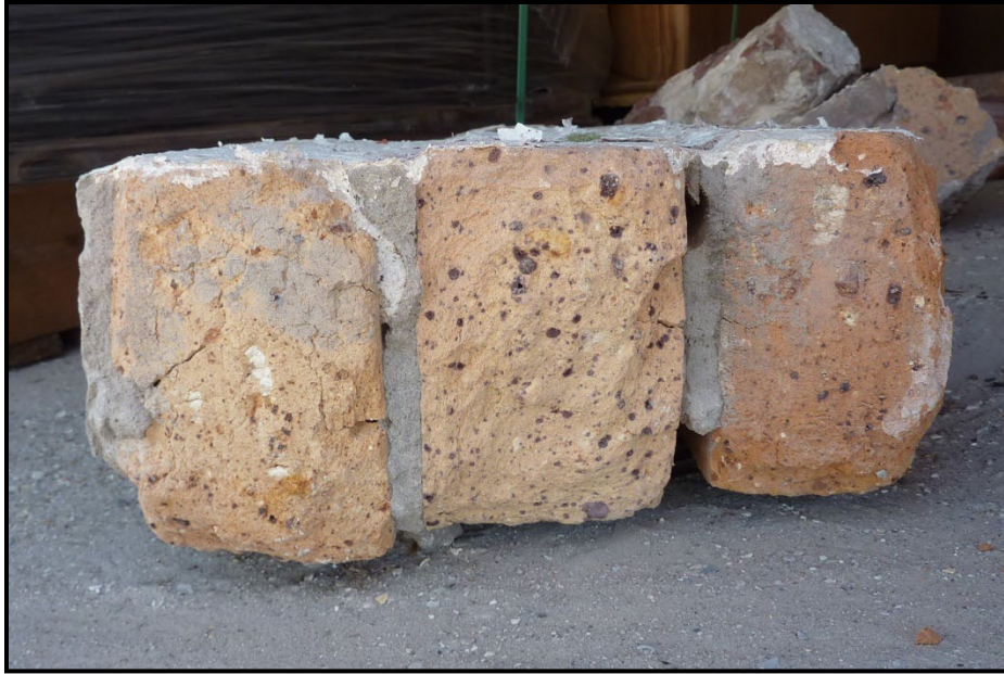
Photo 7. A segment of the oil house wall comprised of common brick and intact mortar covered with paint on the exterior surface. The exterior surface is located on the top of the pictured segment. Note the variations in brick color.
