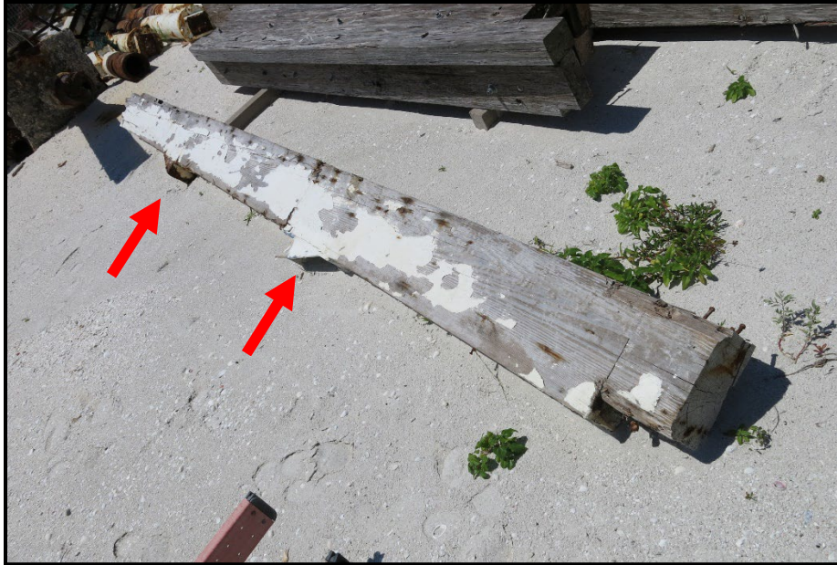
Photo 18. The wooden girder with intact mortise and tenon joints. The right end of the girder is intact; however, the left end of the girder in the photograph has been broken. The red arrows indicate the location of the metal brackets on the bottom of the girder. The mortise and tenon joints are located along the top of the girder.
