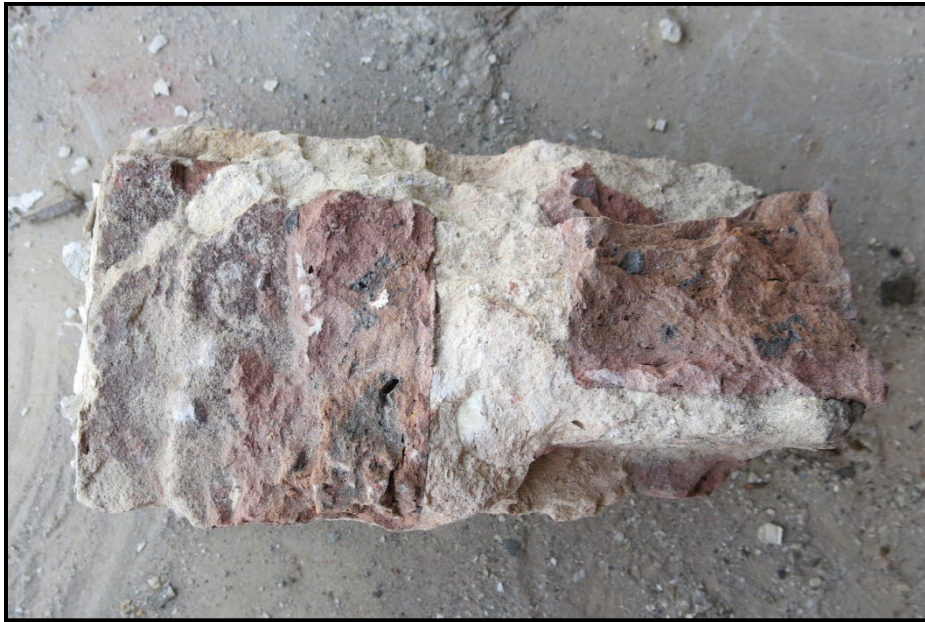
Photo 8. A segment of the oil house wall comprised of common brick and intact mortar covered with paint on the exterior surface. The exterior surface is located on the left side of the pictured segment. Note the variations in brick color.
