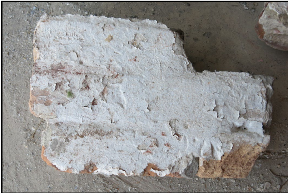
Photo 6. A segment of the oil house wall comprised of common brick and intact mortar covered with paint on the exterior surface.
