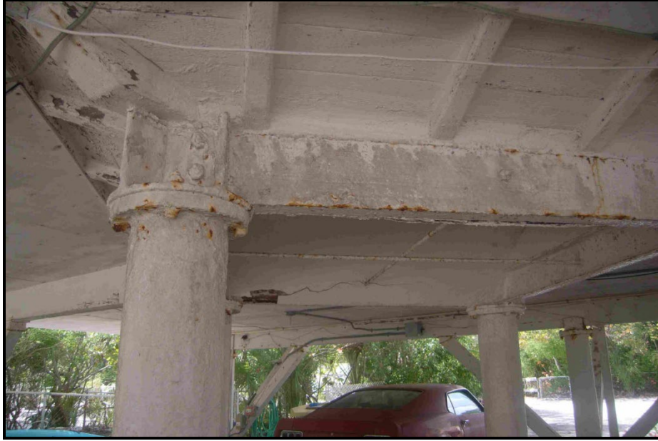
Photo 27. An example of the metal girders in situ beneath the Keepers' Quarters resting on metal support posts (FMSF n.d.).
