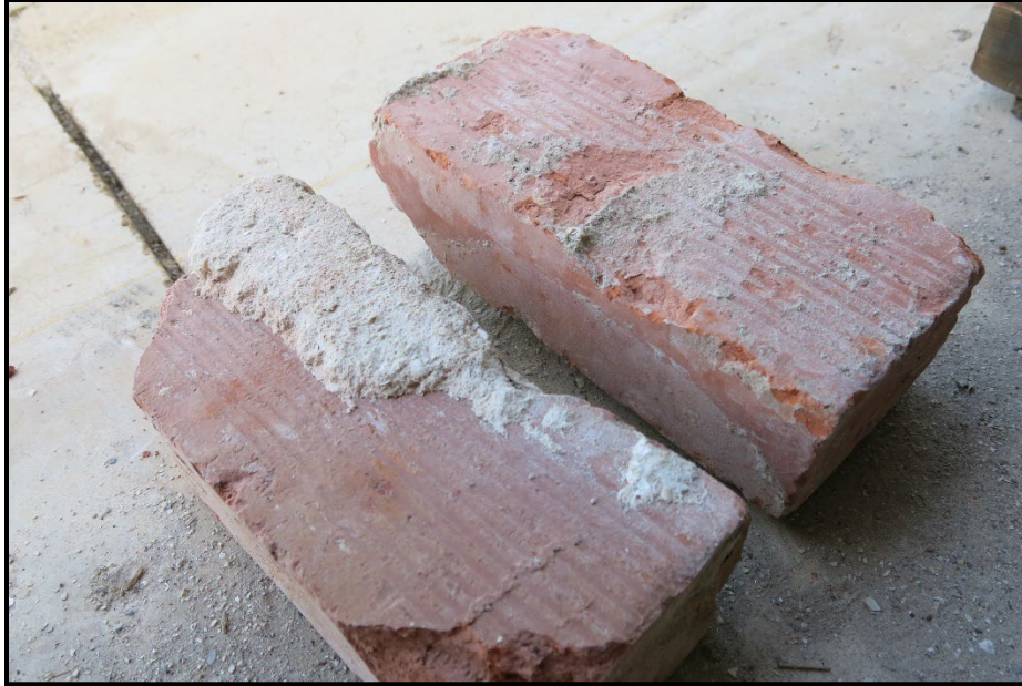
Photo 11. Examples of face brick (striated) identified within the relocated rubble pile. Intact segments of the cistern walls can be seen in Debris Pile – Group No. 2 below.
