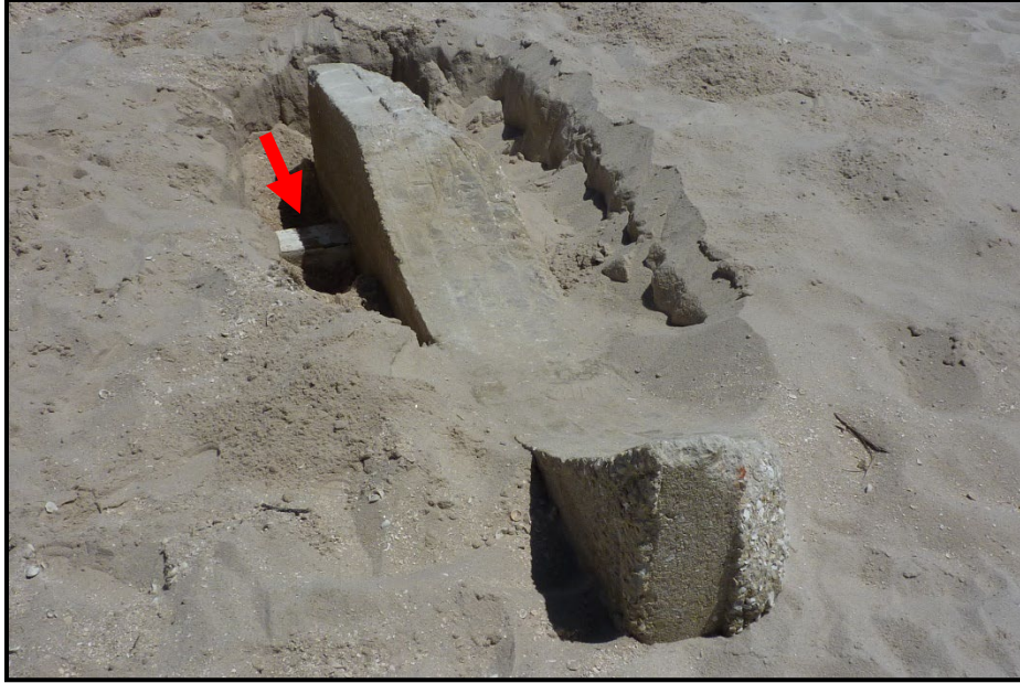
Photo 28. The concrete footer, partially buried beneath the sand and rotated onto its side by stormwaters. The squared wooden support post for which the footer was laid is indicated by the red arrow. The curved surface is lined with brick impressions from the brick cistern.
