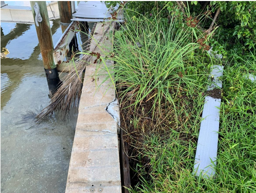
Figure 3. Section of damaged seawall cap
